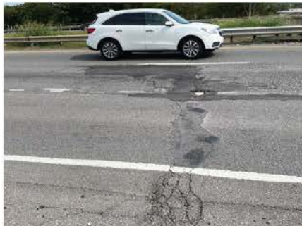
Asphalt &amp; transverse joint damage at approach slab
