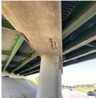
Delamination &amp; exposed rebar at pier cap
